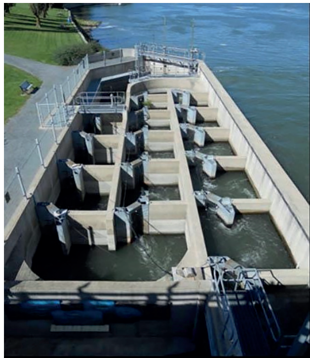
Figure 3. The St. Ours dam on the Richelieu River in Canada has one of the few proven efficient fishways for (lake) sturgeon (Thiem 2013)
