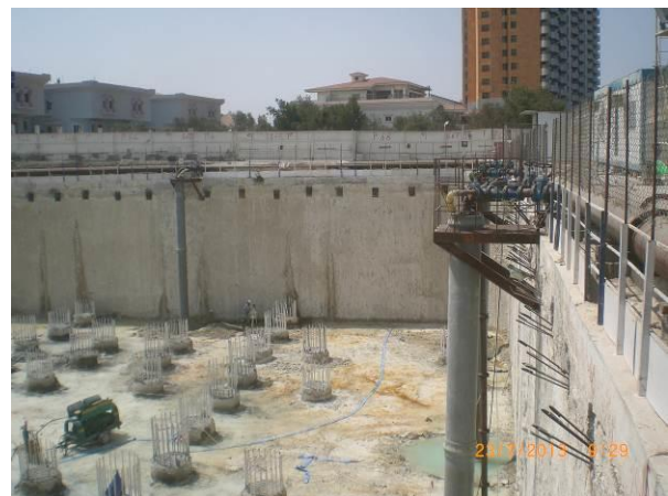
Figure 24 Water Drainage in Operation
